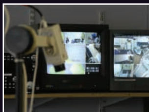
Receipt and despatch of all items is carried out under video camera
